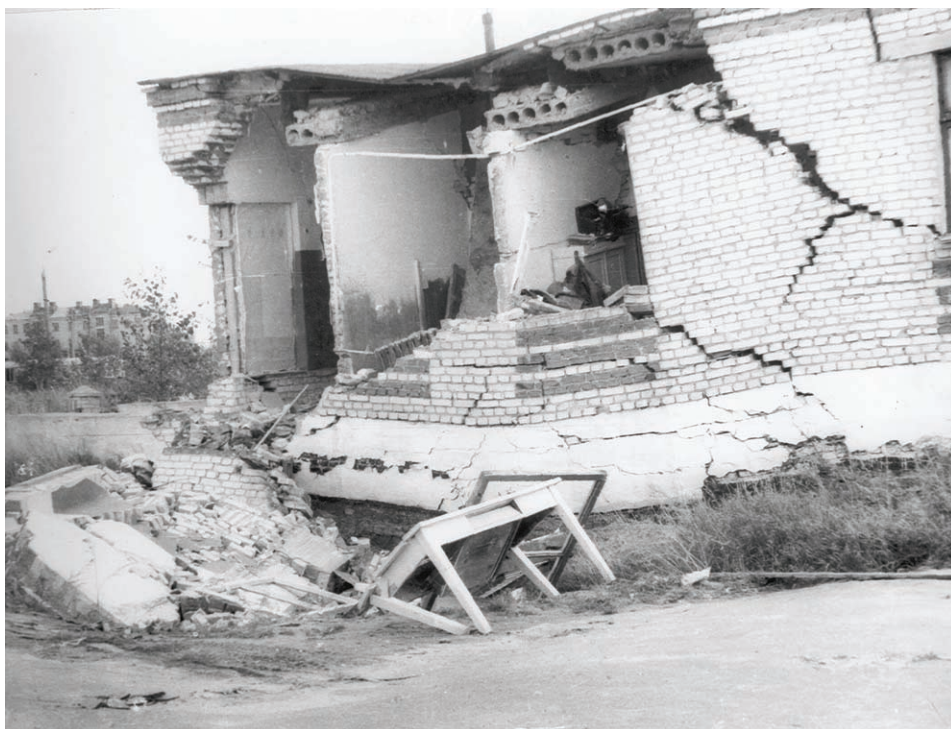
Figure 2. Karst collapse ( d \approx 12 m) in Dzerzhinsk. One more example of building without constructional antkarst protection (Russia), 1970.
