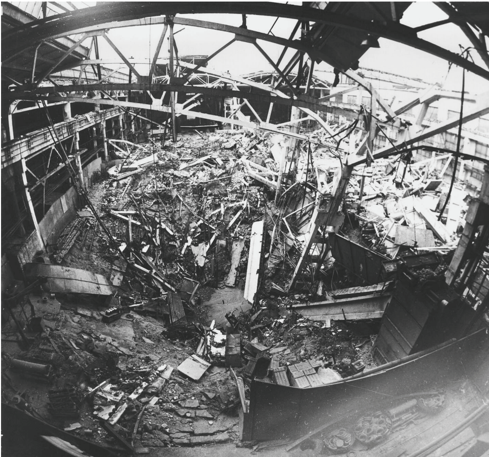
Figure 1. Karst collapse ( d \approx 32 m in diameter) in Dzerzhinsk “KhimMash”. Building without constructional antkarst protection (Russia), 1992.
