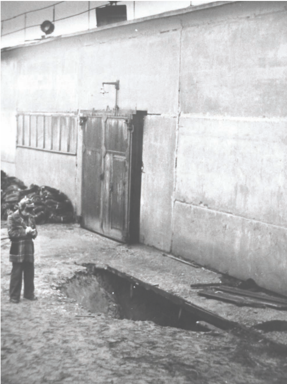
Figure 4. A case of efficient constructional antikarst protection (Russia). The building with a karst-proof foundation sustained a sinkhole d \approx 6\text{m} , (1970).
